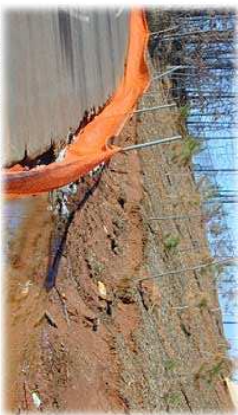
Erosion caused by surface runoff
